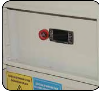
Genel Alarm İkazı General Alarm Warning
